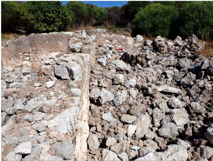
Figure 41. Collapsed wall obscuring ground surface in the Davilak Ruins Complex – Northwestern Section
