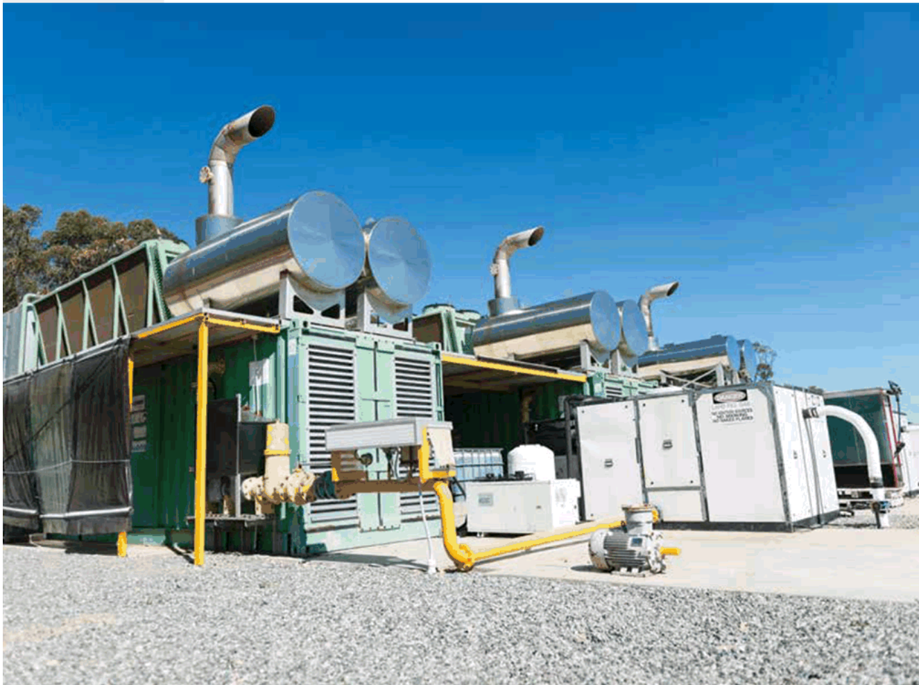
Top: Operations Centre Above: Henderson Waste Recovery Park, methane power plant
