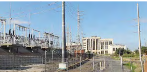
FIGURE 47 - SWITCH YARD AND POWER STATION
