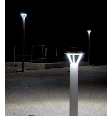
Bollard and overhead lighting
