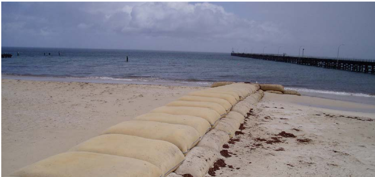
Offshore breakwaters and groynes are examples of hard passive interim protection measures. This groyne example is made from geotextiles. Groynes can also be constructed from rocks to extend their design life. Offshore breakwaters can interrupt open views of the ocean, and groynes can create a barrier along the beach.
