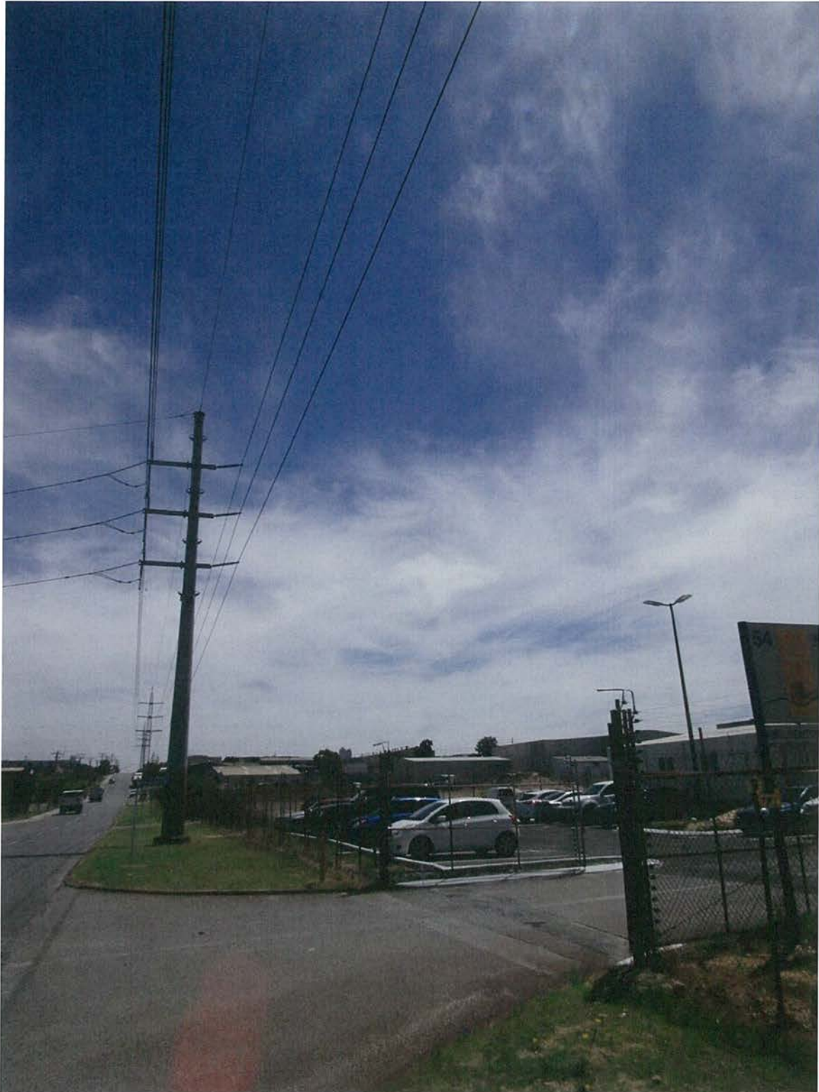
Overhead power lines emanating from a nearby substation dominate the streetscape (source Aurecon)
