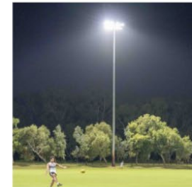
New floodlighting to support sport activities, varying between 300 lux for cricket fields, and 100 lux for soccer fields
