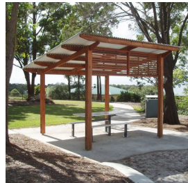
Addition of one shade shelter and picnic amenity, next to cricket nets
