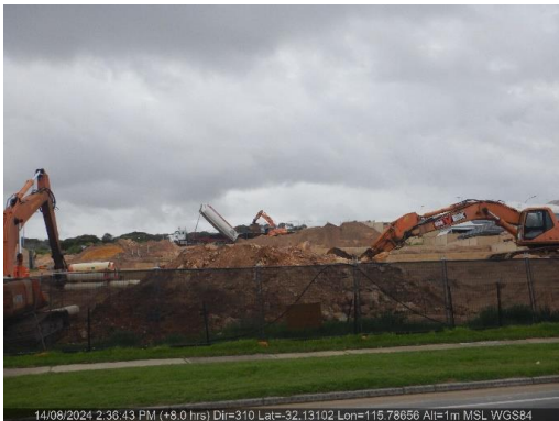
Photo ID: Photo 3 Looking at the major earth works south of the subdivision site.
