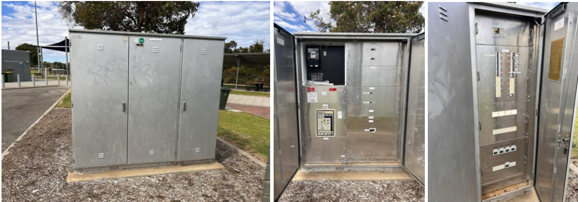
Image 4 - Existing Site Main Switchboard
