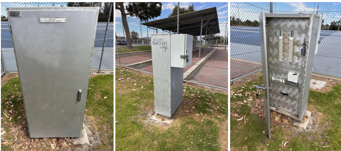
Image 6 - Existing Netball Distribution Board
