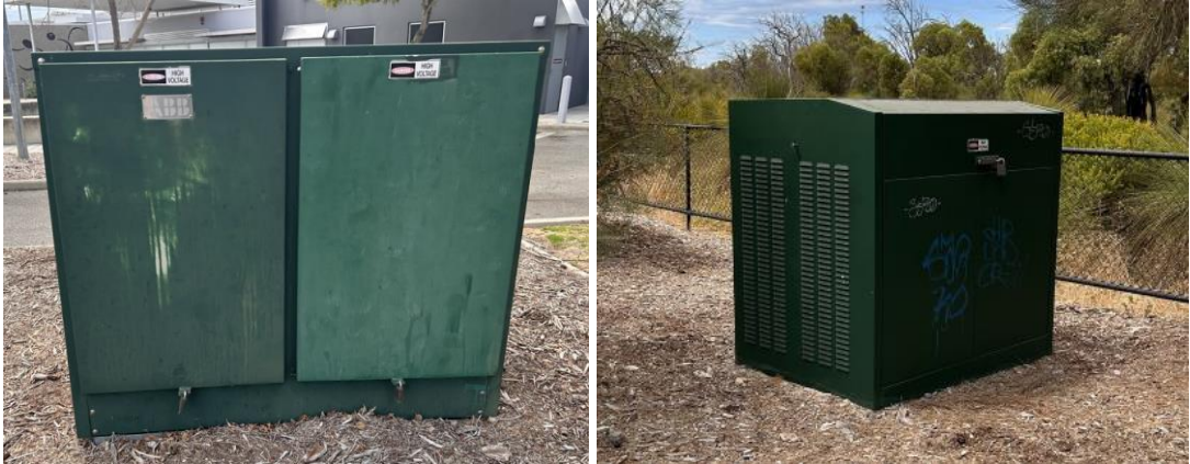
Image 2 - Existing Western Power transformer & RMU
