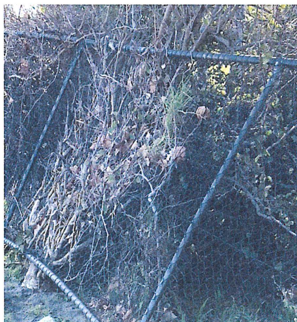
Damaged localised fencing
